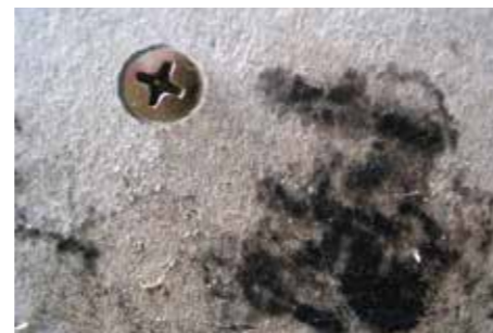
Mould growing on the face of an alternative wet area lining.
